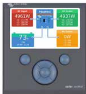
Color Control GX, showing a PV application
